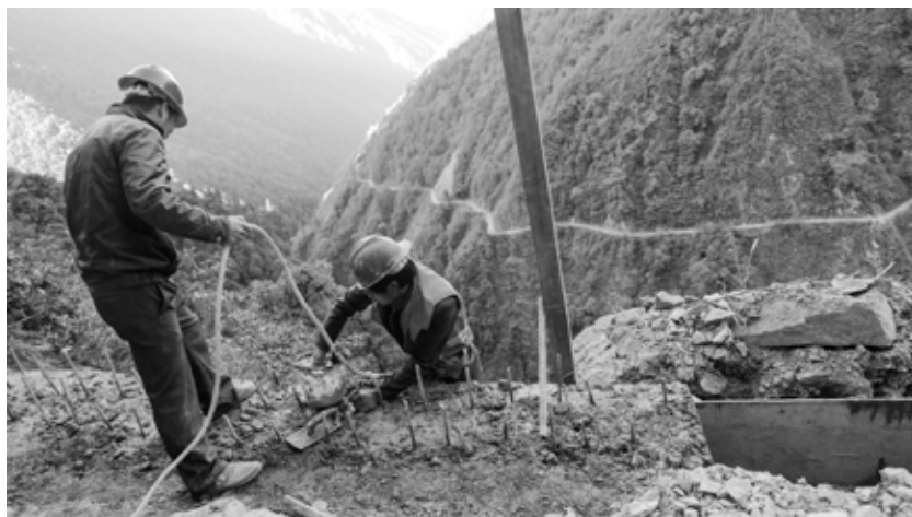
Figure 9: Construction work on the road between Gongshan and the Dulong Valley (picture by the author, 2016)
